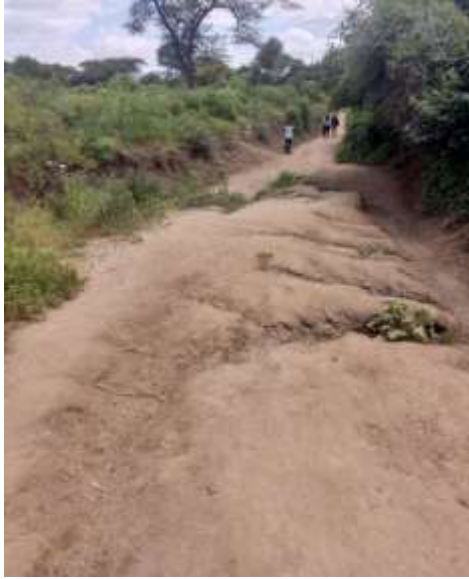
Figure 23: Road turned into a river course 21.9"E alt 748m)
